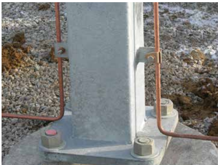
Substation earthing riser
