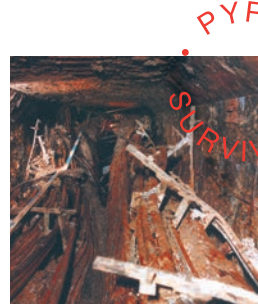
Pyro MI survived in this power station fire
