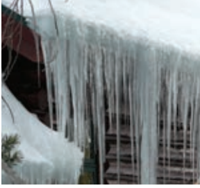
Unprotected roof and gutters
