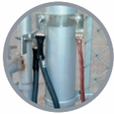
Fence and Gate Jumper Assemblies
